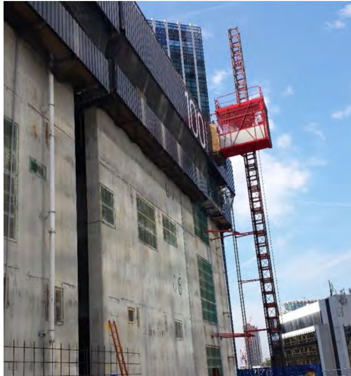
Figure 14. External hoist at 100 BG.
