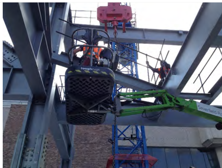
Figure 6. Nature of work may not allow workers to rapidly respond to evacuation alarm.
