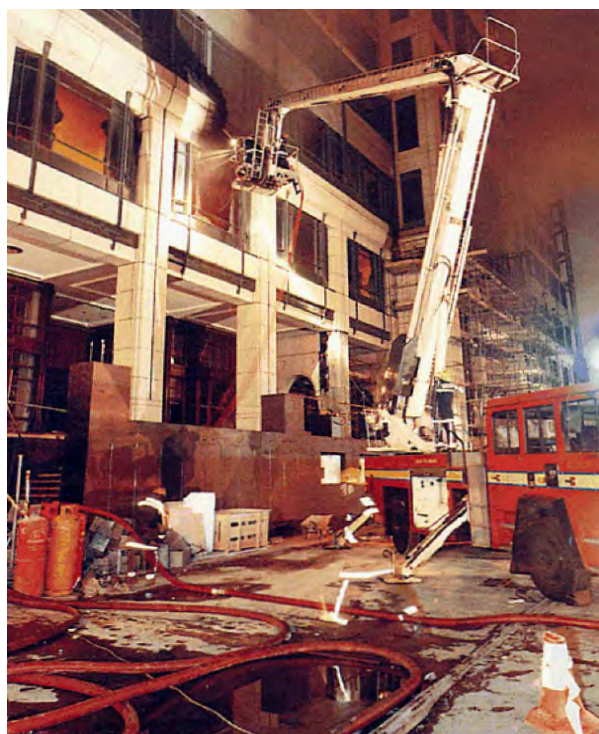
The Broadgate Phase 8 fire, London, UK 23 June 1990 [10]
