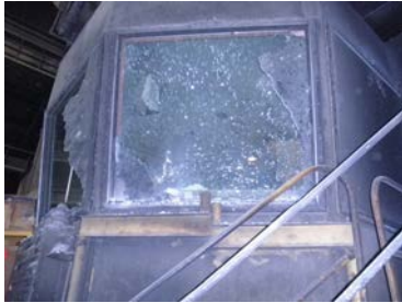
Figure 1: Pulpit Windows Damaged by Explosion
