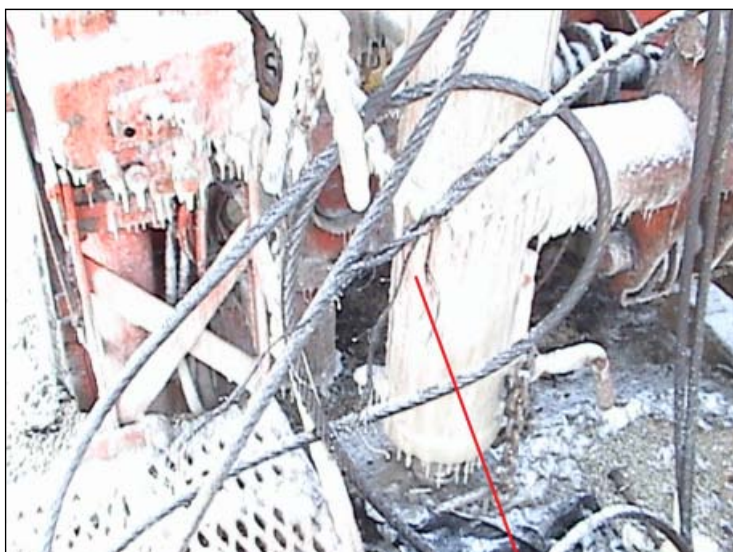
Location of failed 7/8" load line.
