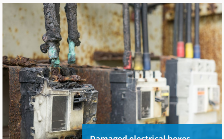
Damaged electrical boxes.
