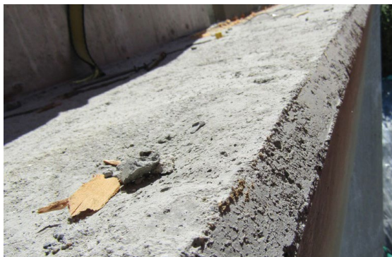
Image 3. Concrete edges can cut lifelines and lanyards.
