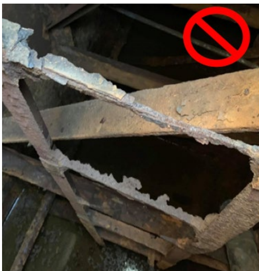
Example of damaged access ladder.
