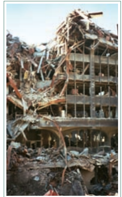
WTC BUILDING 6 PHOTO FROM FEMA
