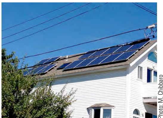
Figure 7.14. Photovoltaic panels on a roof.
