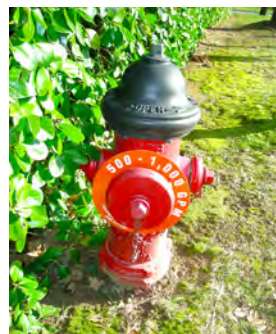
Figure 4.8. A fire hydrant with flow indicator sign.
