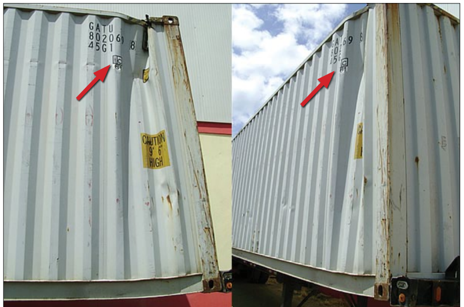
Figure 1: Intermodal container with structural damage.
