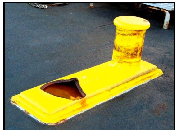
Figure 1. A hollow area under a mooring bitt.
