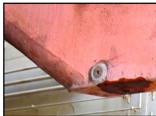
Figure 3. A vent plug indicating leaking product.
