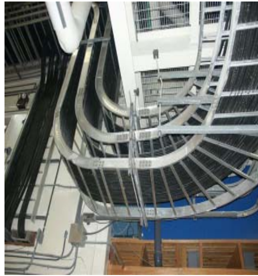
Figure 3. Electrical wires in multiple cable trays.
